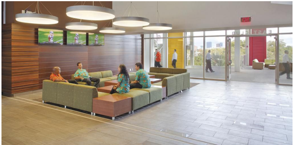
Large buildings such as stadiums need expansion joints for the integrity of the building. But strength and durability can also be coupled with aesthetics and décor, as shown here at the Citrus Bowl stadium in Orlando, Florida. The joint pan incorporates the floor finish, and coordinated seal colors allow the joint to blend right in, which reduces sightline disruption.
