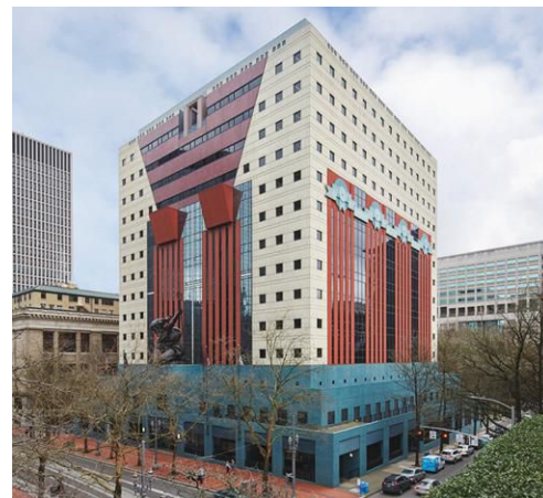
The Portland Building has experienced extensive leaks since its completion, so DLR Group's restoration plan includes measures to better weatherproof the structure.
