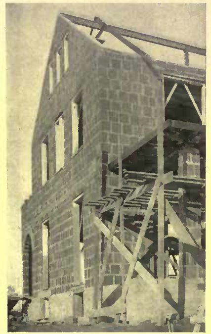
Ready for the roof, which, in this case, is to be of terra cotta blocks held by steel angle beams
