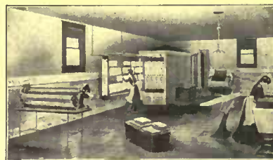
A Modern Residence Laundry Room showing installation of "CHICAGO-FRANCIS" Dryer & Laundry Stove
