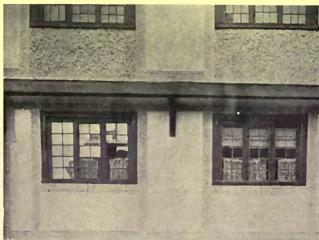
A simpler form of parge work that is more applicable to American needs. The rough panels below the upper windows are pebble-dashed. Note the ornamental bands
