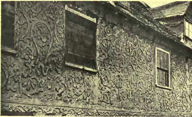
While we would not choose to employ parge work to such an elaborate extent as here, there are excellent opportunities for its use in belt courses and inset panels
