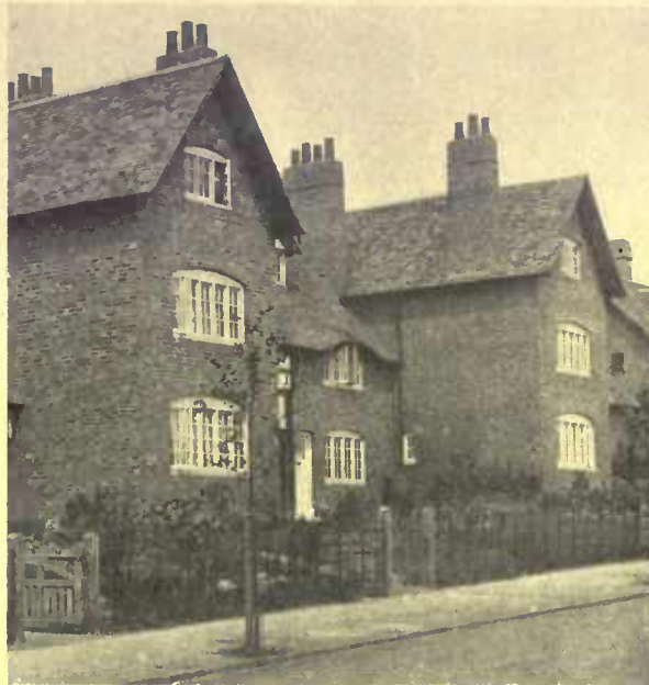
Common running bond in its best form. Every fourth row is one of alternate headers and stretchers to tie the facing brick to the rest of the wall
