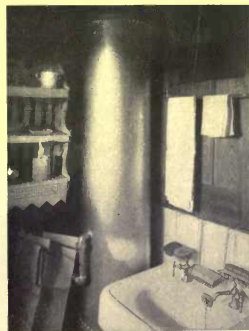
A bungalow bathroom where space is at a premium. The boiler provides the heat necessary on cold mornings and leaves more room in the kitchen
