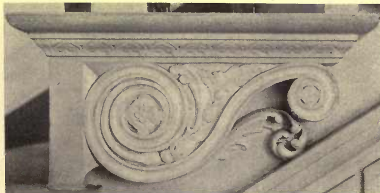
The ends of the stairs in Colonial work were usually embellished with a hand-carved bracket motif, often of great beauty
