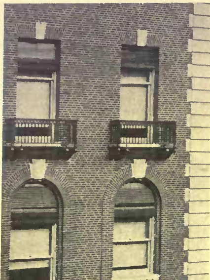
An un-named bond that is seldom seen, giving a curious diaper pattern. It consists of rows of headers and stretchers alternating with rows of stretchers alone, the latter breaking joints in alternate courses. Sperry, York & Sawyer, architects
