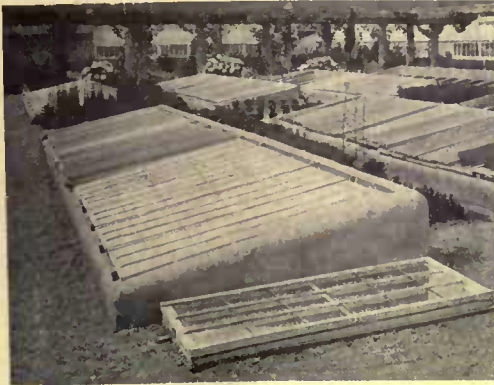
Probably the most economical and serviceable structure is one made of concrete. With some boards, cement and sand, you can make one yourself
