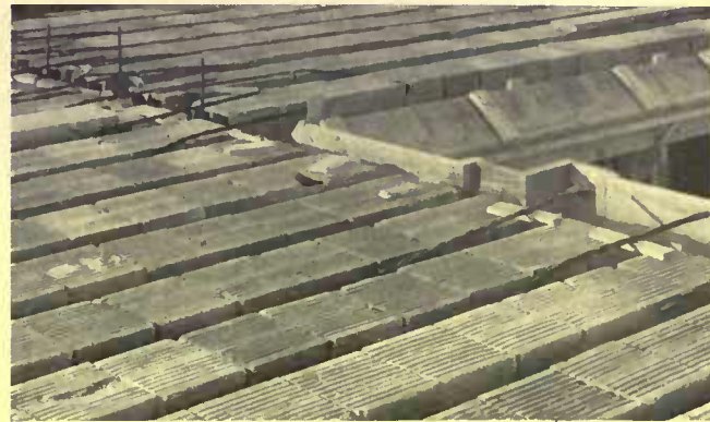
One form of fireproof floor construction. The terra cotta blocks are held up by a temporary support, with spaces between the rows. In these are laid reinforcing bars, over which is poured concrete. The finished floor on top of this may be of tile or of wood
