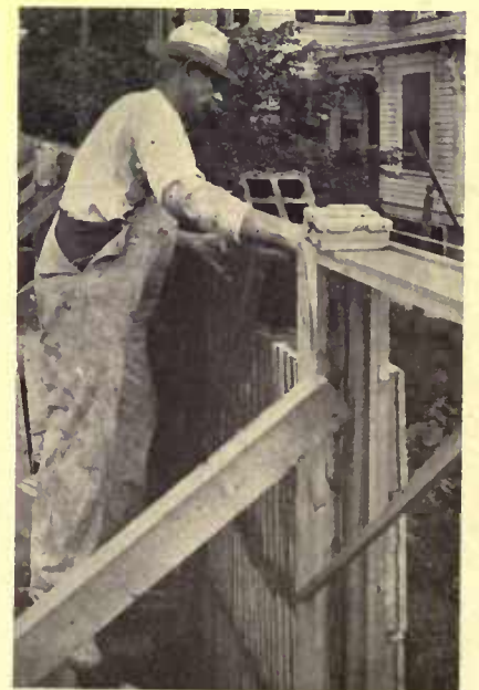
A special form of block is made for the window jambs to bring the wall out to an even edge
