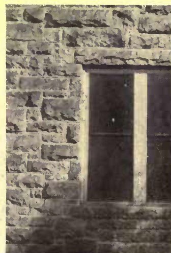
Squared pitched-face stone laid as broken-course ashlar. The edges only are straight
