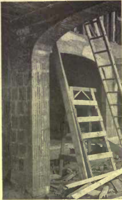
The interior of a hollow terra cotta house, showing a concrete arch resting on the block partition
