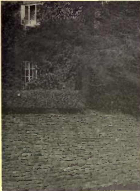
A dry wall—that is, laid up without mortar. It is suited only to garden walls
