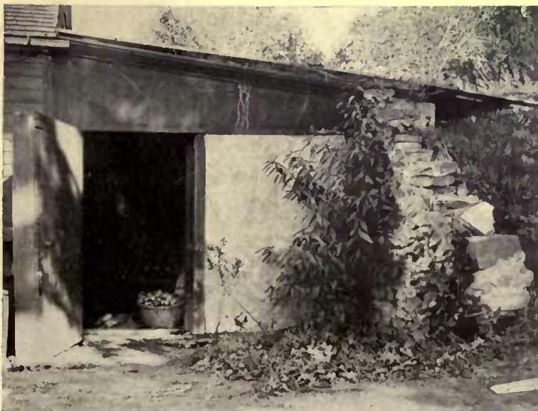
A cellar built into a hillside. Its walls are air spaced and by keeping things dry, cool and well ventilated decay is prevented
