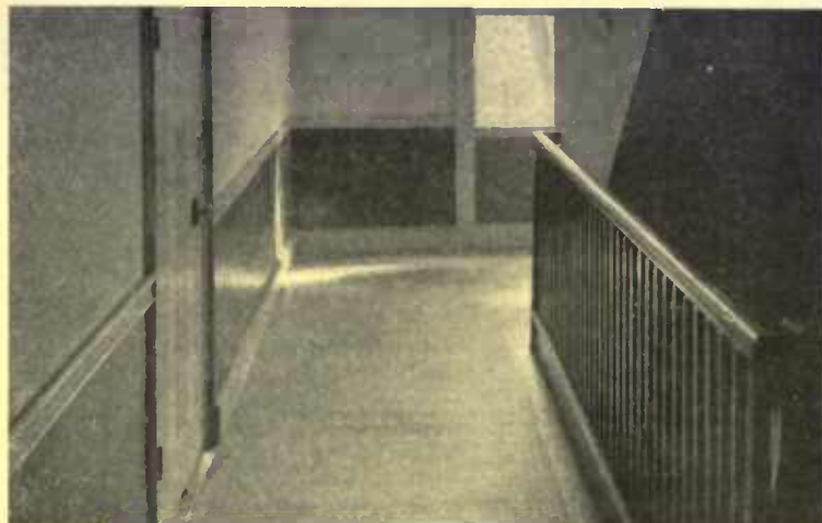
Even the old floor yields to this treatment. Smooth off, apply a filler and proceed as directed
