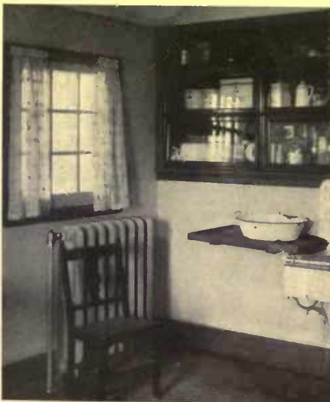
The improved vapor systems bring the steam in at the top of the radiator. It flows steadily and obviates all "knocking in the pipes"
