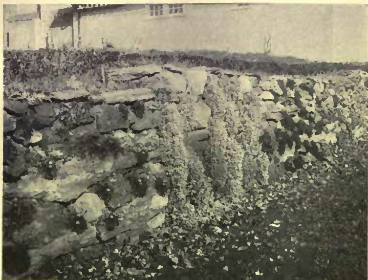
In the cracks and holes of a rough wall, creeping plants take hold and grow vigorously
