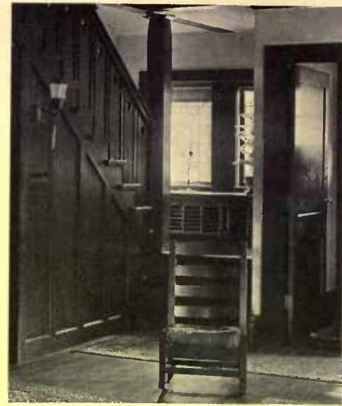
The steam radiator is not placed where necessity demands, but can be located where it can heat incoming cold air
