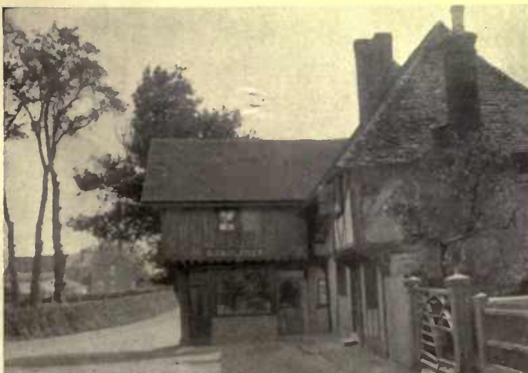
Brick was frequently used for filling in between the timbers, as here in the herring-bone pattern. When poor brick and other miscellaneous filling was used, it was plastered over
