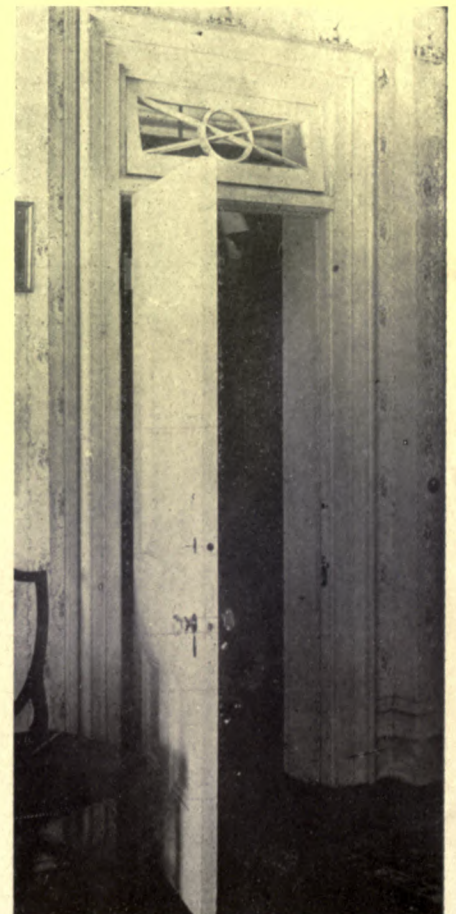
The slight decoration in this transom adds the note necessary to complete the impression of a Colonial room
