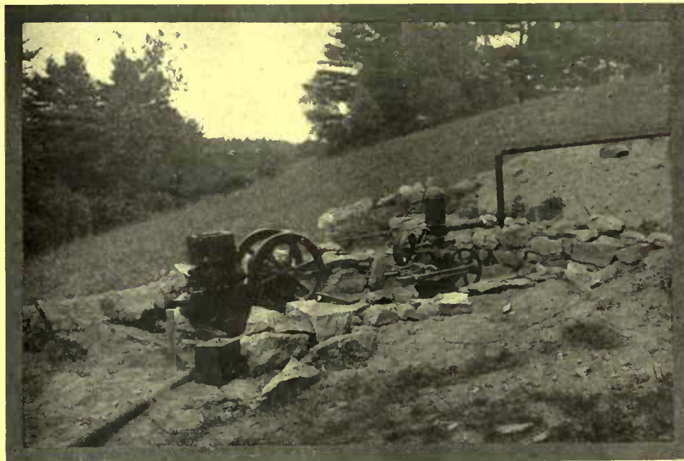
The pump and gasoline engine for forcing water into the spraying pipes were installed on the sloping ground near the pond
