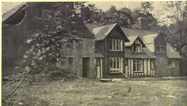
While the west wing was being worked the east wing was occupied and the owner had the pleasure of being at hand to watch developments
