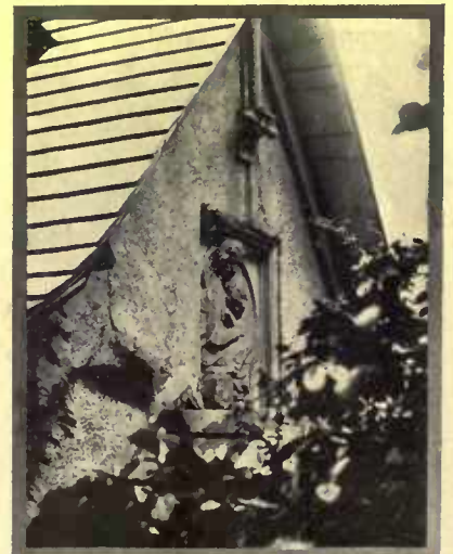
A useless outhouse window filled with an inserted concrete medallion
