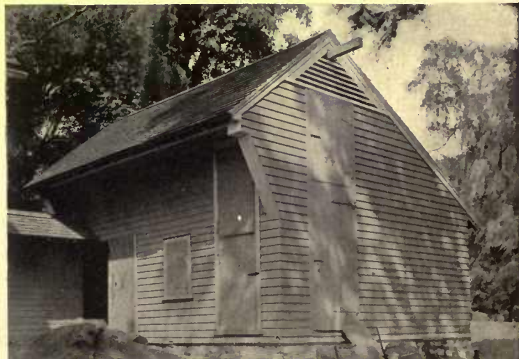
Some sort of ventilation, such as fixed slats or open spaces under the eaves, must be provided to carry off the moist air
