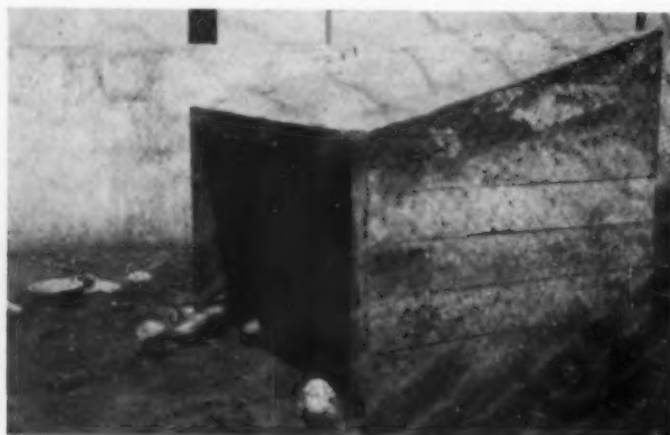
Utilitarian throughout, concrete was employed even in such a small detail as the making of a chicken coop, rat proof and easily kept clean
