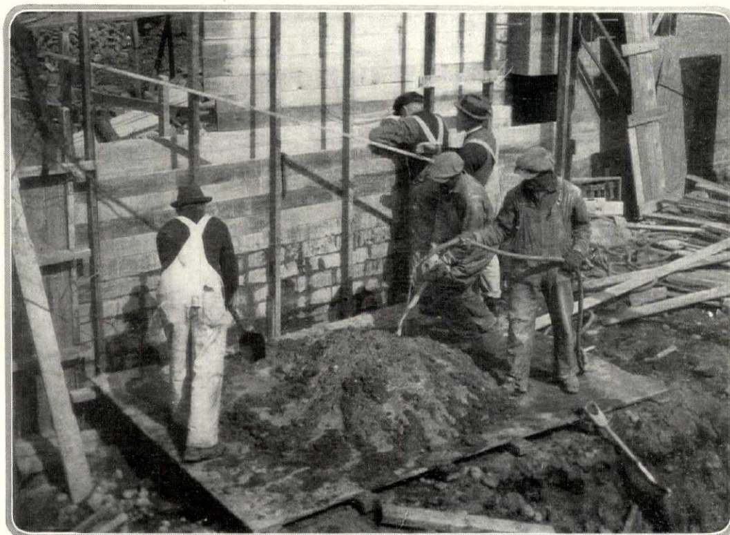
The actual mixing of the concrete preparatory to filling in the forms is here shown. Clean sand, cement and gravel or broken stone are the ingredients of concrete
