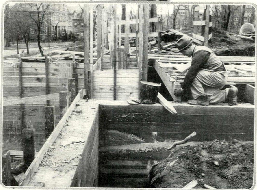
The appearance of the foundation wall after the forms have been removed may be seen at the right. The joists for the first floor are being set in place
