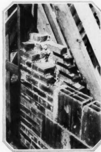
Views of partially completed hollow tile walls. Around some door frames, brick as well as tile is used in the construction. The hollow tile is to be coated with stucco
