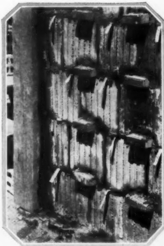
At the extreme right, workmen are constructing a hollow tile wall. Projecting metal strips and wood blocks are left to bond the tile to the brick and half-timber exterior
