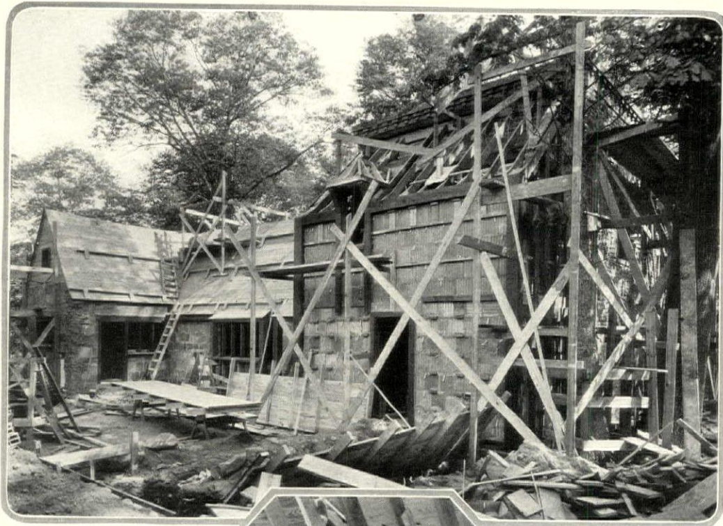
(Above) Sheathing is being laid on the roof of the main portion of the house. This sheathing aids the shingles, which will next be applied, in roof insulation
