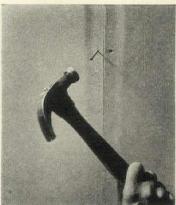
A. This fireproof wallboard, available in large lightweight sheets is first nailed to studs
