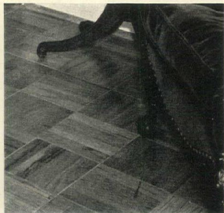
Beveled edges on this block floor conceal any slight irregularities in alignment caused by an uneven sub-floor. E. L. Bruce
