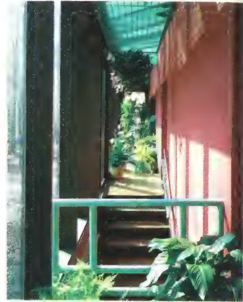
Stair from ground to living level seen from short catwalk. This is Trombe wall's air space.
