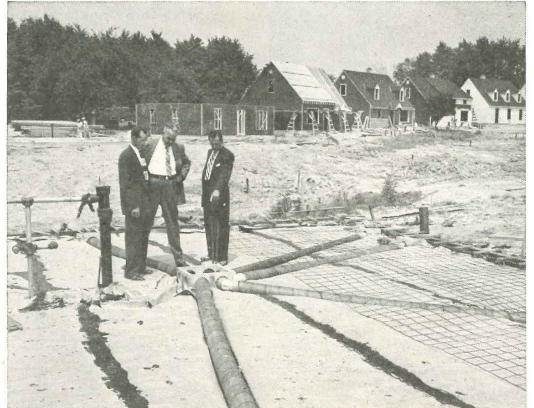
At this stage the moisture barrier has been laid over gravel fill. Six-inch ducts are now resting in trough made by lower channel. As slab is poured, concrete flows entirely around the air duct, forming 2" covering.
