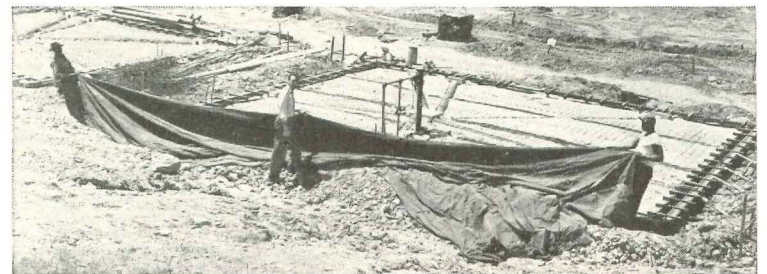
If there was any chance of rain, tarpaulins were spread over gravel at night to keep out moisture before next day's slab pouring. Six by six reinforcing mesh is used.
