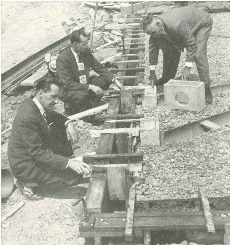
Foundation walls and slab are poured in one operation. Portable wood form serves as outside wall. Inside wall is 1" x 12" insulation board of asphalt covered glass fiber with a 1/2" x 8" gypsum stiffener. Removable paddle dams (held by Dvorak in foreground) serve as form spacer as well as helping to control the pouring operation. Inspector Scheel, right, is pointing to precast register boxes. This corner of the house is the living room where two registers are close together under a 6' window.
