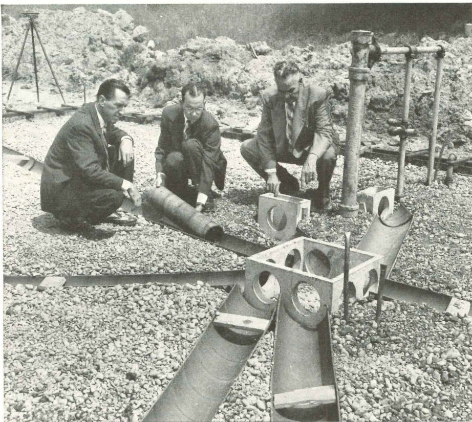
The 10" fiber channels before moisture barrier is spread. Precast plenum pit is made by local burial vault firm. Left to right: Dvorak, James Martin of Warm Air Assn., City Heating Inspector John Scheel. A wood cover keeps concrete out of plenum.
