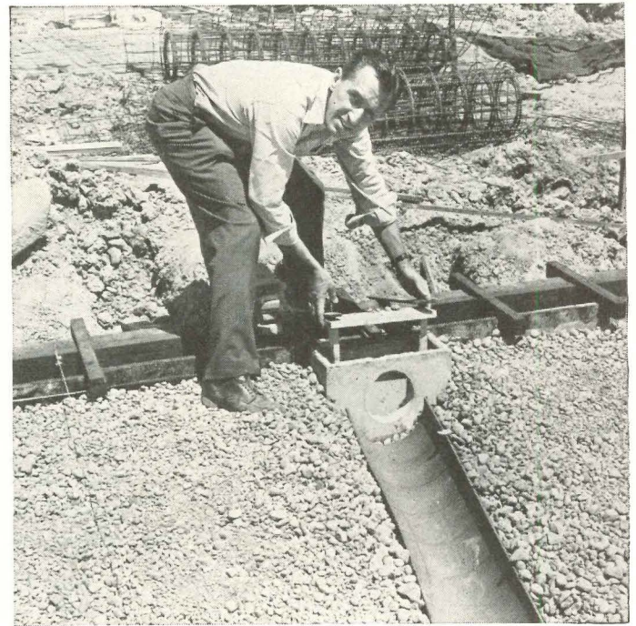
Wood stools, like the one held by Dvorak, are inserted in precast register boxes to keep out concrete and all other rubbish while construction is going on.
