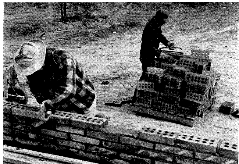
Great economy comes from 6" thick through-the-wall bricks which are not backed up by masonry block as is customary in all-masonry house construction. Furring strips are fastened to wall to which are nailed dry-wall panels backed with reflective insulation. Bricklayer's helper gets $2.27 hourly base pay.
