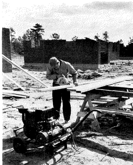
Gasoline generator provides power for cutting rafters, interior partitions and other necessary lumber. Carpentry labor costs $475, lumber $640, trim and windows are $360.
