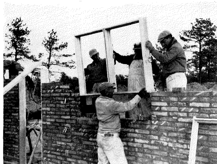
Windows slide easily into position because slot in each brick forms T & G arrangement with frame. Foreman works inside of house, makes sure of window and door locations, gives general supervision to two houses under construction.
