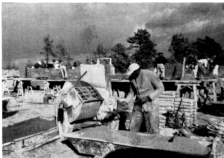
Nearly two houses per day are now built by 17 bricklayers who use so much mortar that one man spends all his time at this mixer. Fork lift also moves this equipment from house to house. Cement and sand cost $45 per house, bricks $105 per M plus $40 delivery. Job is fully unionized.
