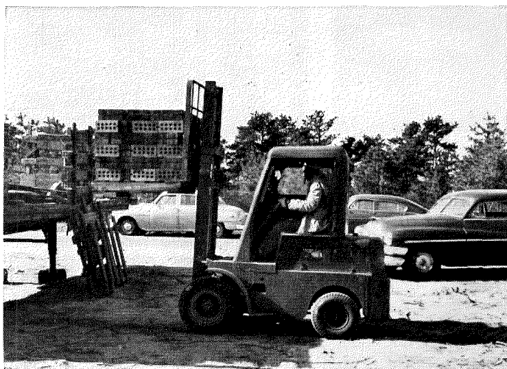
So fast were the 17 bricklayers that the builders had to buy this Clark fork lift to speed up brick handling. It cost $3,000 secondhand, but saves $40 per day by eliminating two men. One man now unloads truck and distributes loaded pallets. House has 3,229 bricks plus 244 cinder blocks.
