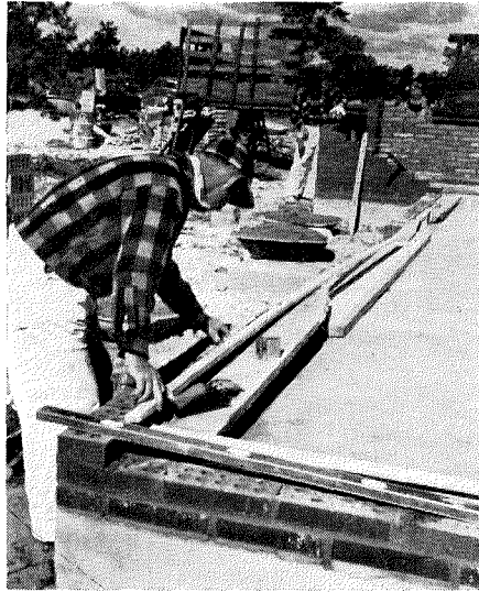
Door and window positions are marked by this wood template. Conventional footings and slab cost builder $525. Sheet-metal ducts for warm-air furnace are embedded in slab.
