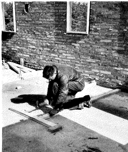
Conventional wood-frame partitions go up quickly once the brick exterior walls are finished. VA financing was so attractive to a local bank that no premium was asked for.
