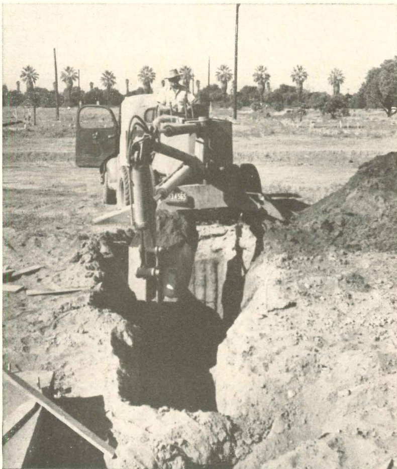
Truck-mounted power shovel digs one septic tank cavity per hour. Such power equipment helps Hadley-Cherry deliver houses from 90 to 100 days after starts.
