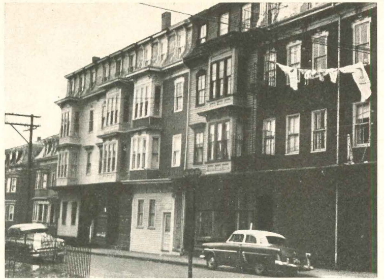
MARKED FOR DEMOLITION in renewal block shown in "before" and "after" photos on p. 45 is the left end of this four-story frame flat. Court has banned new occupants in extreme left bay until owner, 78, repairs it.
