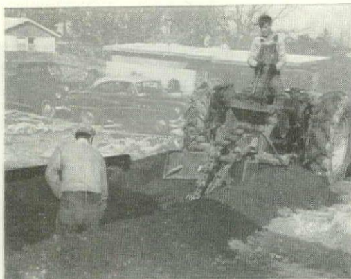
Lightweight fiber sewer pipe quickly follows trenching machine into the ground, is coupled to the next piece with a tight-fitting ring connector. Not as resistant to damage as some other types of pipe, the fiber material is usually buried far enough below the ground to be safe from such crushing blows as those of a heavy delivery truck.
