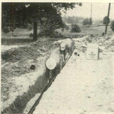
Perma-Line is installed quickly. Several 5, 8, or 10-foot lengths can be joined, then laid into the trench and tapped onto the line.
