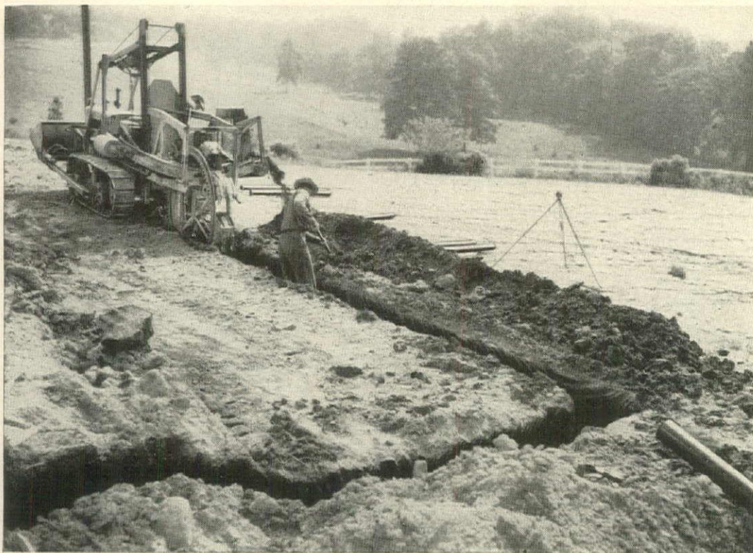
A land-drainage installation of perforated Perma-Line pipe on the J. L. Shannon estate near Detroit. Photo Courtesy Superior Tank Company.
