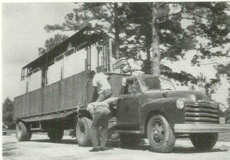
8 AM: Truck arrives at site with complete first load: six sections of steel frame, 16 steel trusses, 34 galvanized steel, paint-grip birdstops, plywood for roof, two gable ends, exterior gypsum for wall sheathing, concrete panels to go over windows, metal spline connectors and nails.
