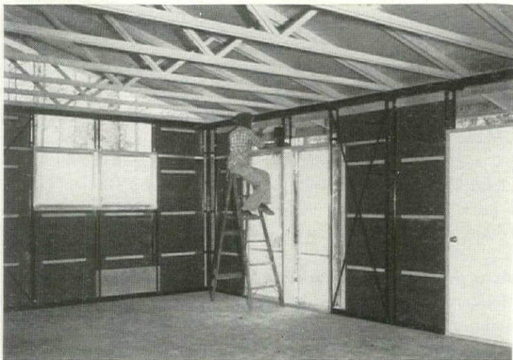
11:45 AM: Workmen put finishing touches to exterior: here birdstops are fastened to trusses over windows where concrete or metal panels will be inserted. Within 15 minutes, before lunchtime, house will be ready for mechanical trades and interior partitioning (see pp. 142-143).
