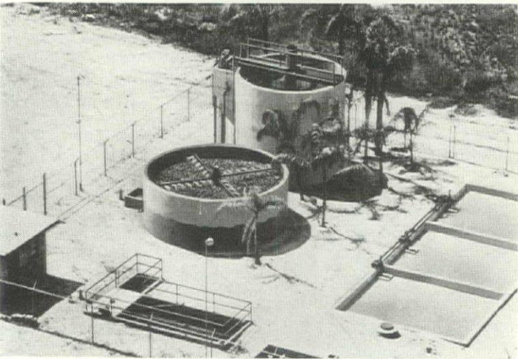
Primary treatment plants sometimes suffice for sewage treatment and of course greatly reduce costs. This plant in Center, Colo. serves a population of about 2,000. Unit includes upper compartment for clarification and separate sludge digester.
