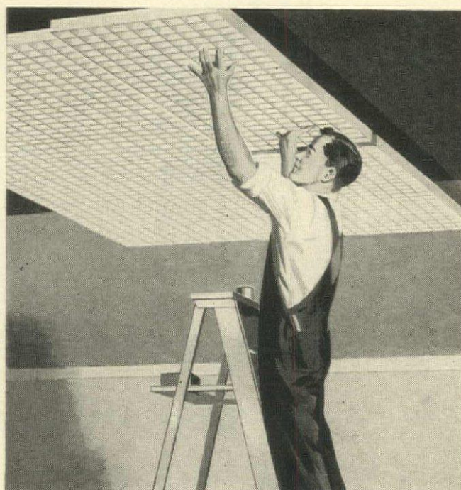
4. ALUMINUM GRID CEILINGS made with Kaiser Aluminum boast lasting good looks, long life without maintenance. Their bright, modern appearance helps attract customers, brightens a store's reputation.
