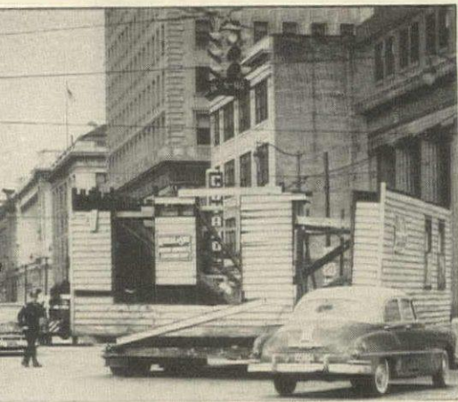
Moving the cut-apart houses through downtown streets gave Operation Demonstrate a chance to show public what was going on, provided many newspaper photographs.
