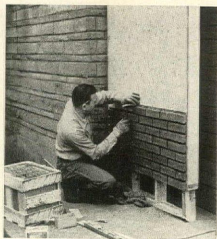
Level courses are nailed to plywood demonstration panel; two nails per brick.
