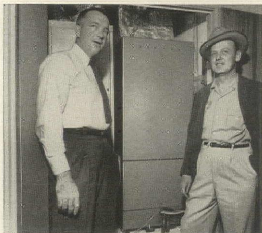
Mr. Thomason and Mr. Lunt beside the installation of a 3-ton Gibson unit. Even on hottest Texas summer days this unit, charged with "Freon", maintains a cool 68° indoor temperature.
