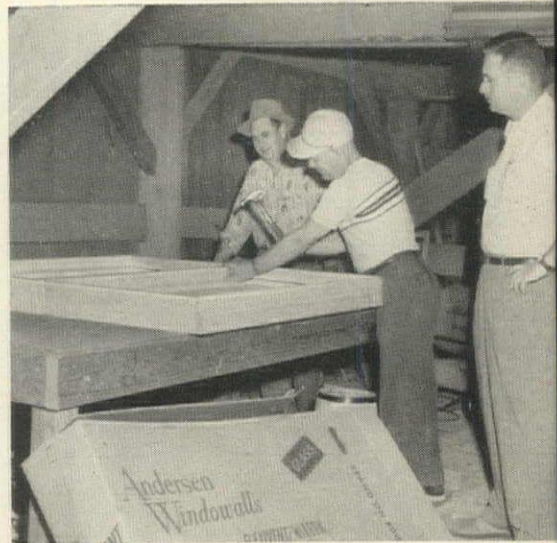
Assembly of Flexivents for an Archer project. "The pre-installation assembly of units is a big factor in expediting our building schedules," reports Mr. Archer.
