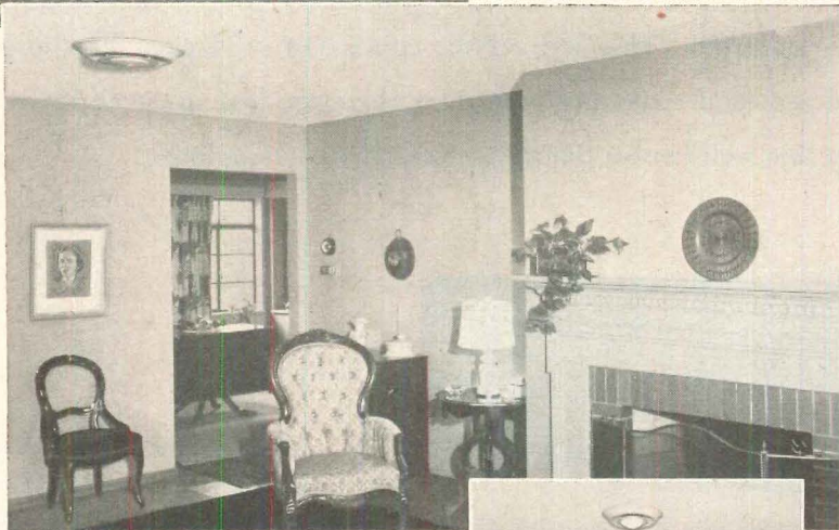
Living room has two Kno-Draft Diffusers. Air distribution system and fan-coil unit are located in attic. The condensing unit is at rear of house.
