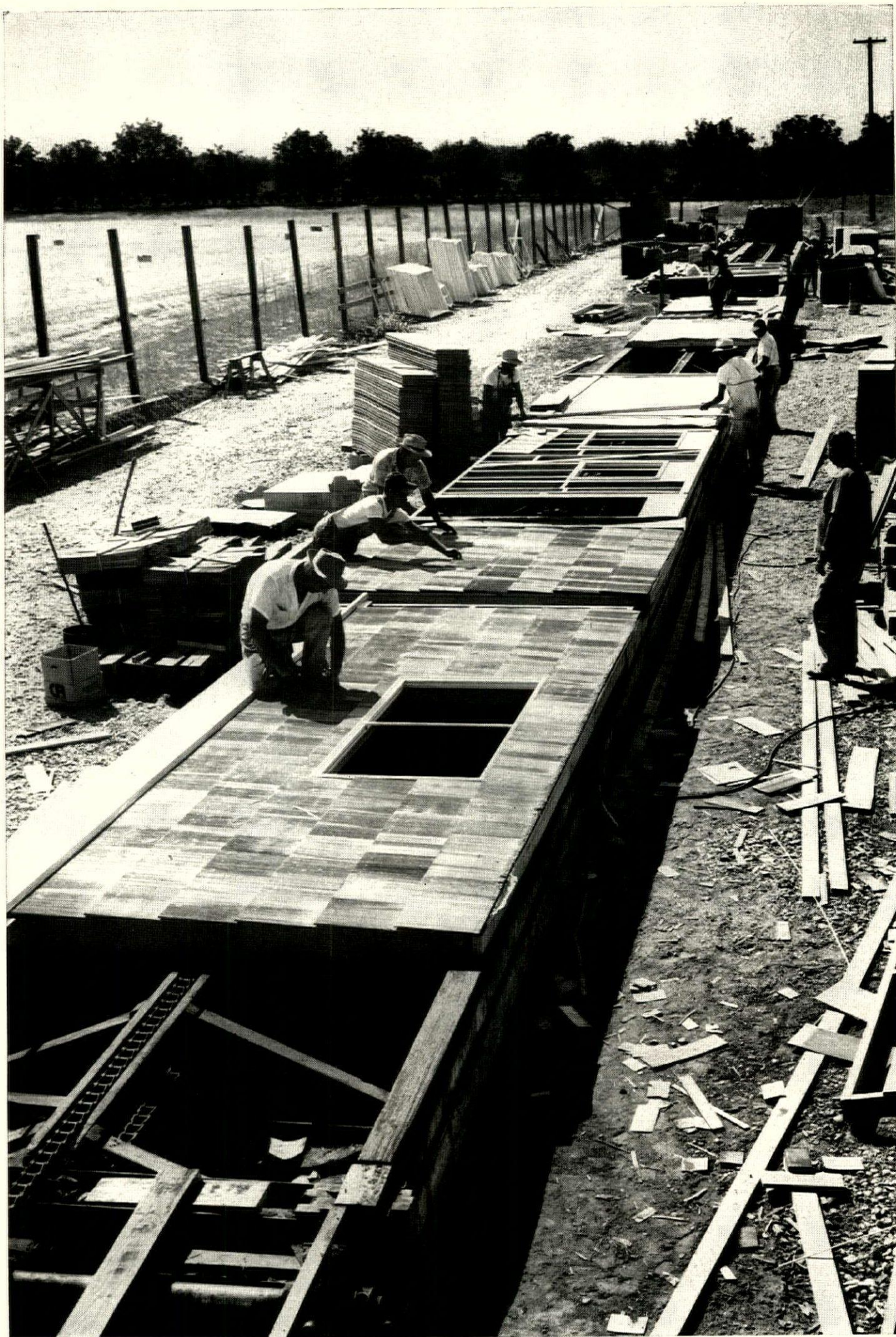
OPEN-AIR PRODUCTION LINE sits on permanent concrete foundation. Panels slide on wooden rails, are pulled along by drag chain
