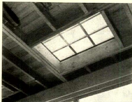
SKYLIGHT rests on framed-in well of 2 x 10's. Bands between blocks are aluminum tees. Headers are doubled front and back.
