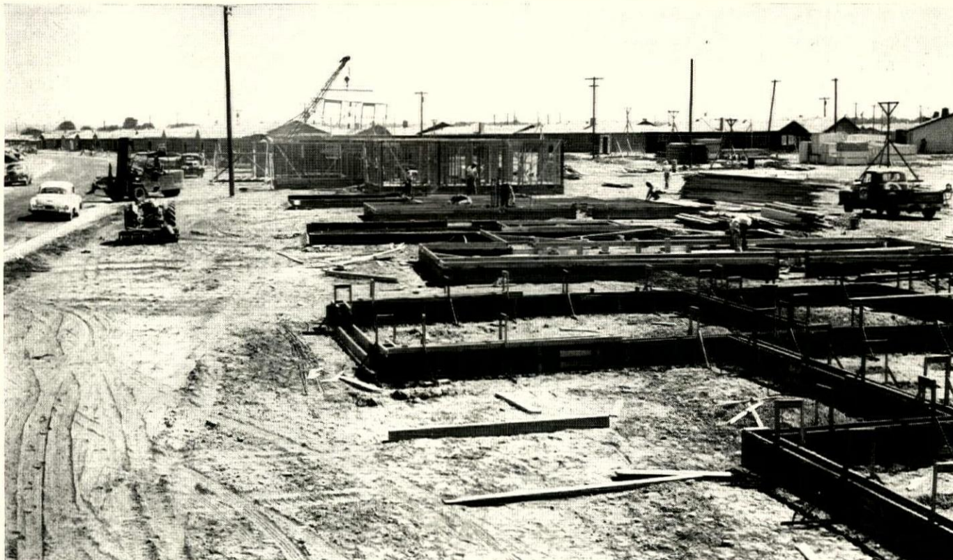
AT THE SITE. Here crane is lifting interior partition into place (rear) while plumbers and subflooring men work on house in middle distance.
