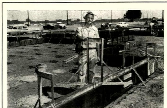
COST-CUTTING DIVIDEND: Foundation templates, designed by Jacobson himself, have completely eliminated stakes and ties. He figures this saves about $30 a house. In two hours, three men can set up the 50 templates and 16" high form boards for foundations of a 1,600 sq. ft. house. On Rancho Cordova's generally level ground, the foundations stop short of the top of the forms, making it easy to set sills. Each set of welded steel templates cost $500, but Jacobson has built over 800 homes with only two sets. At least ten Sacramento builders have borrowed the idea. /END
