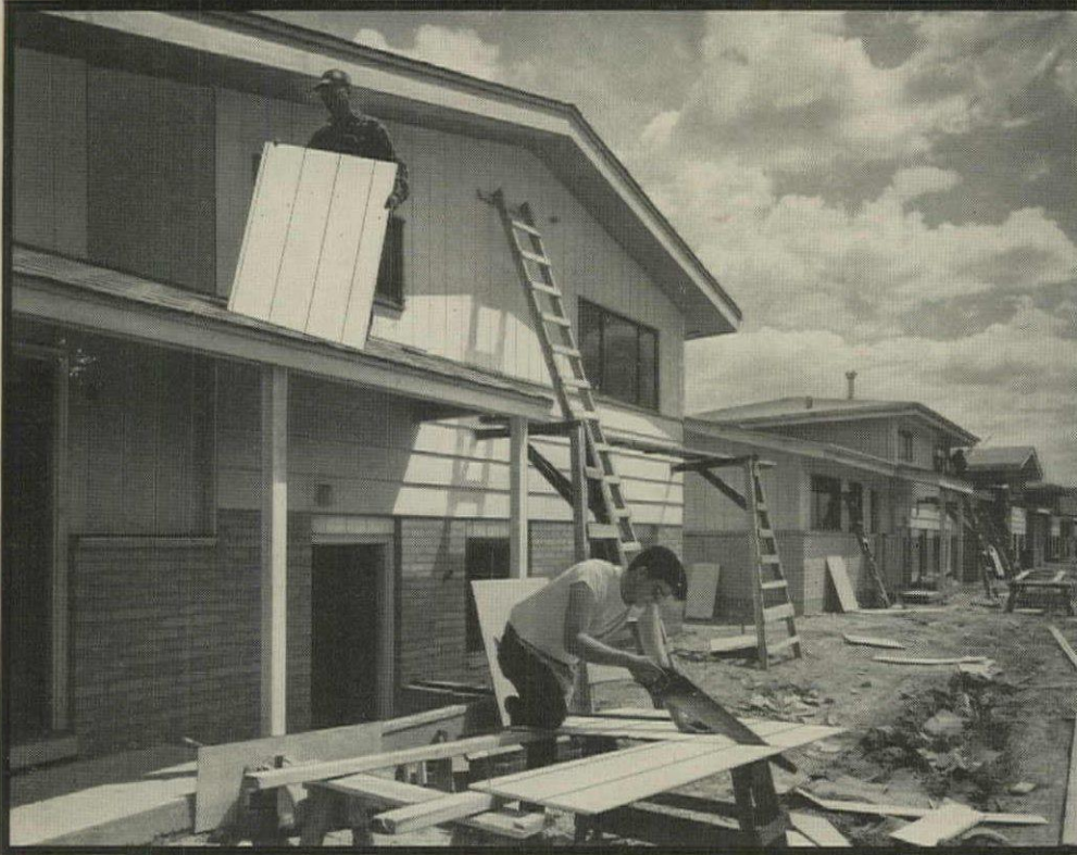
Speedy application of Insulite Primed Siding—both horizontal boards and vertical grooved panels—is seen in recent photo above, made at new Lincolnwood area of Park Forest.
