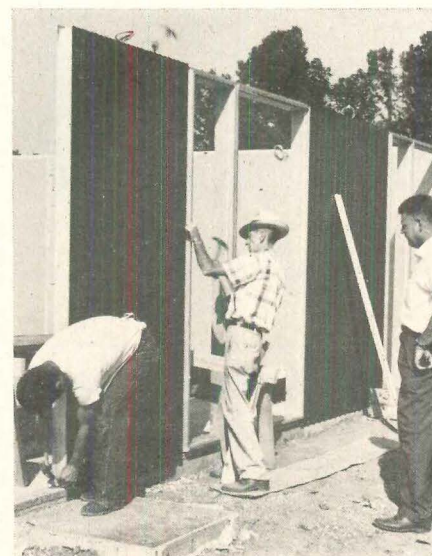
Wall panel edges are toenailed to sill before next panel is placed. Sash bucks are nailed to joint spline and panel.
