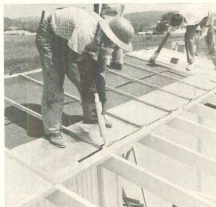
Edge of trellis opening in roof is caulked and weatherstripped before batten-seam sheet roofing is placed.
