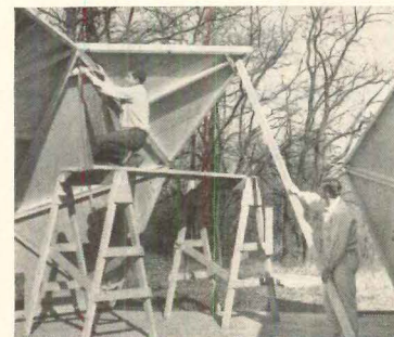
6 Temporary bracing is needed as erection approaches dome closure. Mid-bracing 2x4s in triangles stop short of corners to leave bolting room.
