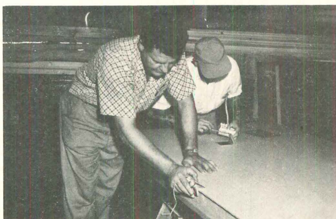
Final step is to glue prefinished interior skin to panel framing. Base outlet box picks up Romex cable in panel and special beveling tool puts miter on panel skin edge for V-joints.
