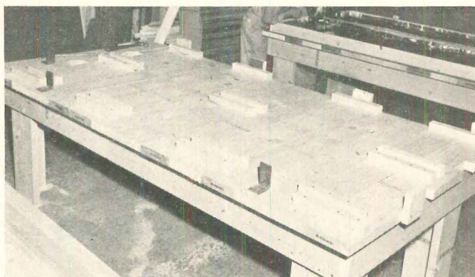
Jig table speeds accurate assembly of panel. Table can be built of 2x8s for $40 to $50. Blocks position framing members, metal brackets serve as stops for placing skins.
