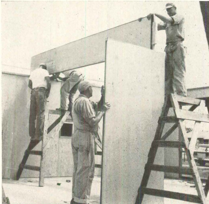
Panelized girder sections are light enough to be manhandled into position. Male end (above) joins female end of next section to make joint over bearing partition.
