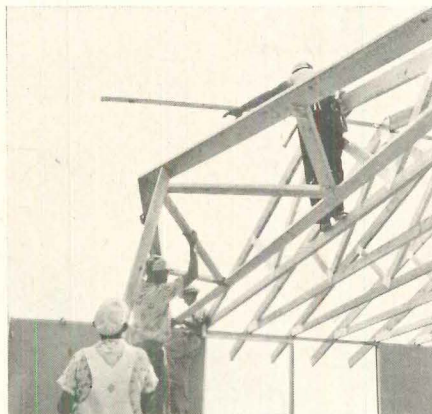
Trusses , W-type with big 2x6 top chord, are positioned by hand. Truss connector is H-Brace nailed from one side.
