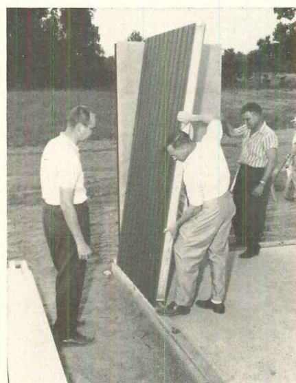
Starting at a corner , wall panels are tilted up, nailed through exterior and interior faces to 2x4 sill plate.
