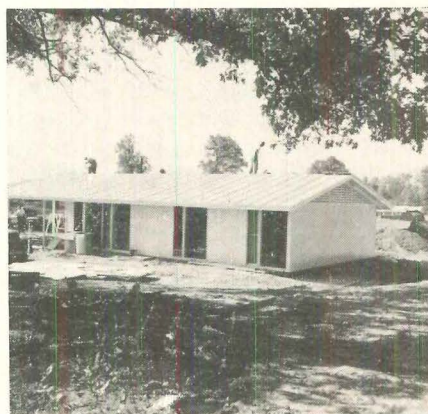
Finished house uses heat-reflecting aluminum roof and light-color exterior paint. Paint is 20-year finish (p 123).
