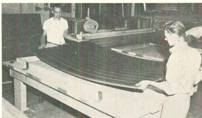
Second step is the fastening of sheathing siding, a hardboard with a board-and-batten surface called (by maker, Masonite) Sunline Siding. Surface can be shop primed for 2¢ a sq ft.
