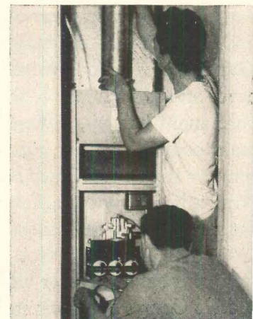
Two-man team installs complete unit and ducts in eight hours. This gas-fired American-Standard furnace, the G.U.B. 75D—delivers 75,000 B.T.U., requires only three feet square. Entire unit is easily accessible for adjustment.
