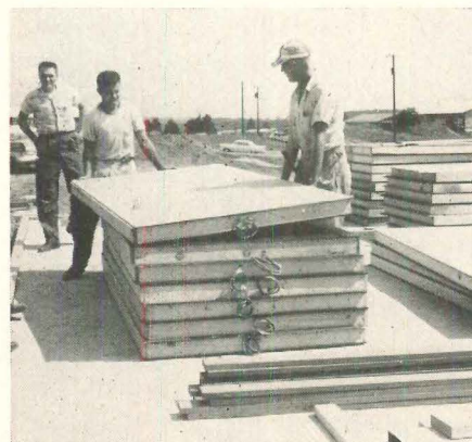
Pre-wired panels , here ready for erection, all have three ft length of Romex cable coiled at top. Cable leads to base receptacle in panel.
