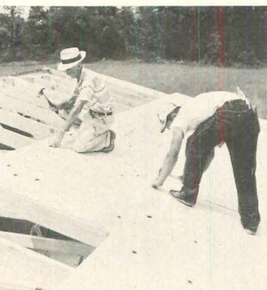
Wood roof-sheathing , in 4x8 panels, closes in house fast. At this point, weight interior partitions go in.
