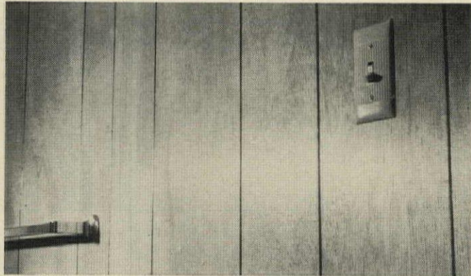
MAHOGANY PANELING with a waterproof sealer is used in the baths. AHG also has cedar paneling in all its kitchens.
