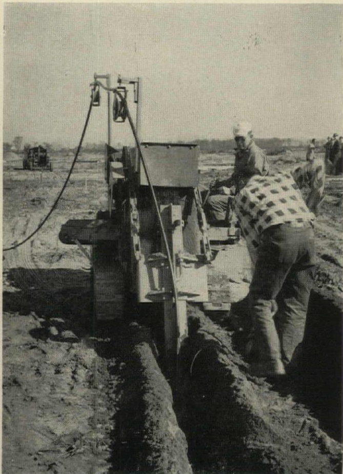
CABLE-LAYING TRENCHER digs 8" trench and lays phone cable in one operation. Metal plate protects cable from trencher's teeth.
