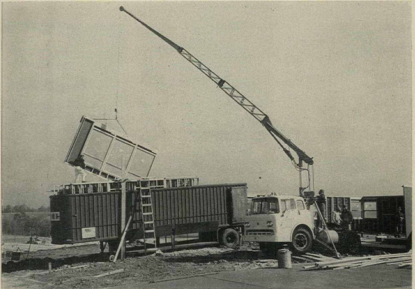
TRACTOR-MOUNTED CRANE lifts window wall from trailer, will swing it directly into position on slab.
