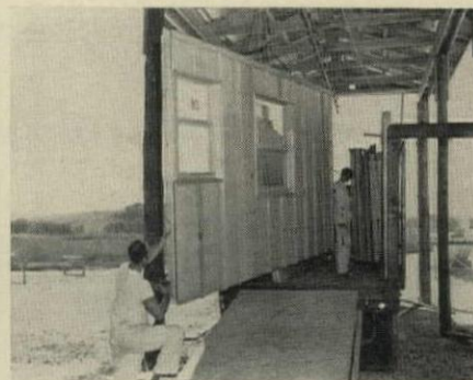
AT SHIPPING DOCK , monorail carries panel onto waiting truck. Soon, panels will be pre-primed before they leave the plant.
