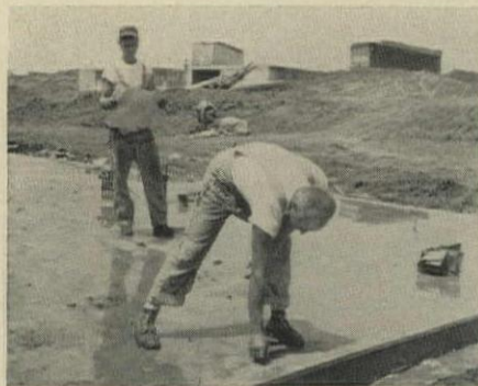
8:00 AM Layout men chalk lines on slab to show panel positions. Trailer loaded with panels is already standing by.
