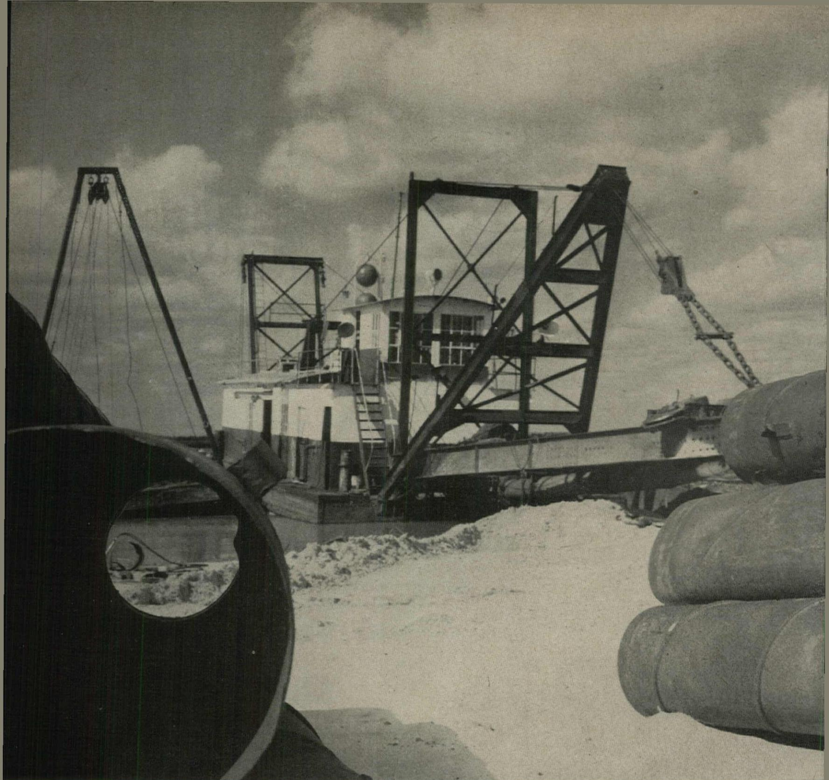
AT PALM BEACH LAKES, big dredges are pumping millions of yards of fill to convert low land into a 5,000-acre residential community.
