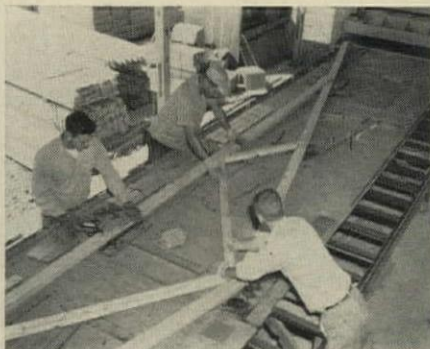
PRECUT TRUSS MEMBERS are positioned in jig on this table. Carpenters tack Gang-nail connectors in place. Then . . .
