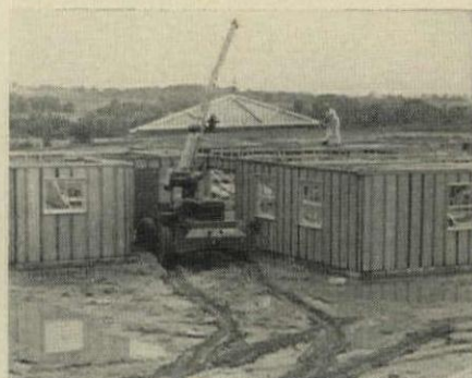
10:50 AM Despite muddy conditions, crane moves quickly into space between house and garage to put gable end in place.
