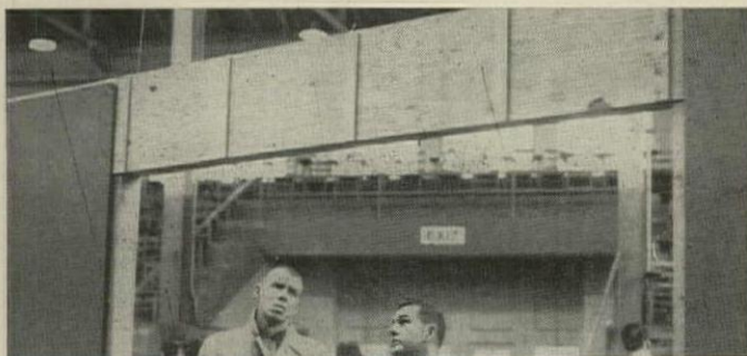
OUTSIDE FACE of headers is plywood. Scabs make up difference in thickness between sheathing and plywood, give flush surface for siding.
