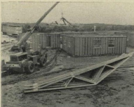
11:00 AM Picking up three trusses at once, crane lifts them high in the air to man waiting to lay them on top plates.
