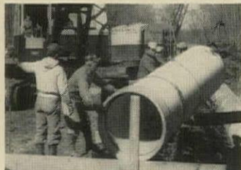
The Sayre Woods South water and sewer systems were installed by Guy Villa & Sons, Inc., Clark, N. J.
