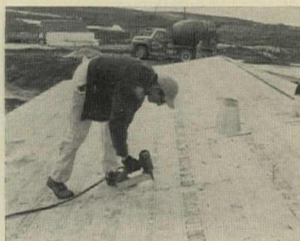
3:55 PM Carpenter completes nailing of roof sheathing in 45 minutes. It was earlier cut and tacked in place by two-man crew.
