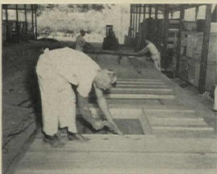
WINDOWS ARE CALKED to get air-tight bond between window and siding. Calking in the plant saves 20¢ a window.
