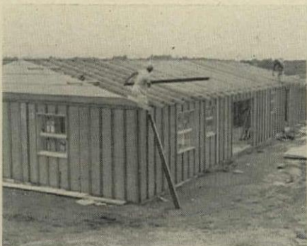
1:00 PM Trusses in place, the house plumbed, one carpenter applies fascia while another is aligning trusses for 2' oc spacing.
