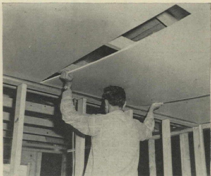
CEILING PANELS are installed from walls toward center of room. Final, center panel is placed by bowing it slightly so ends can slide into SteelFast channel. Ceiling joints are also taped and bedded.
