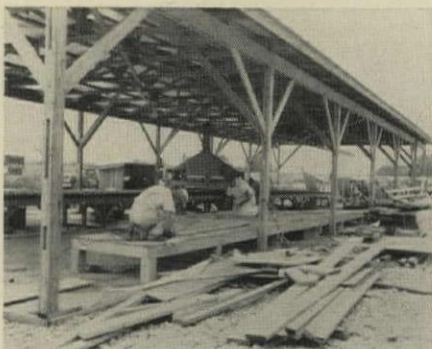
GABLE ENDS are assembled from precut parts on low jig table. Some carpenters used to field work still stand on table to nail.
