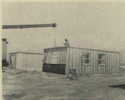
9:05 AM One of the last panels is positioned. Crane holds component while carpenter nails top plate to tie panels together.
