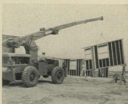
8:45 AM Fifth panel (for rear of house) is brought in position. By now, crane has to move to place parts in right locations.
