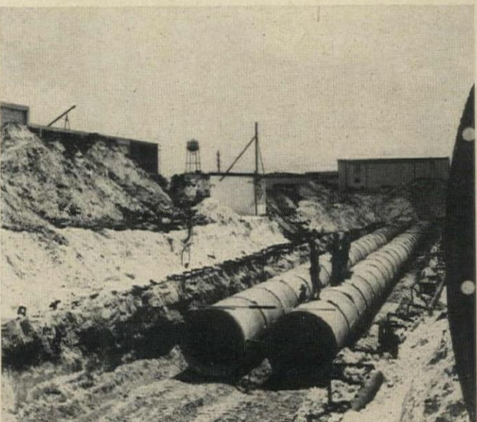
TWIN 60" STORM SEWERS are laid in trench dug by 3-yd bucket dragline. Storm and 20" force-main sanitary sewers are cast iron. Other installations include sewage disposal plant, 28 sewage lift stations.
