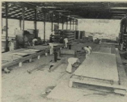
SHEATHING-SIDING is nailed to framing sections on two different lines: one for solid walls (right), one for window walls.
