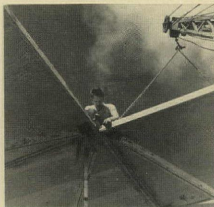
5 Angles and straps tie the units together. Edge beam will surround entire roof.
