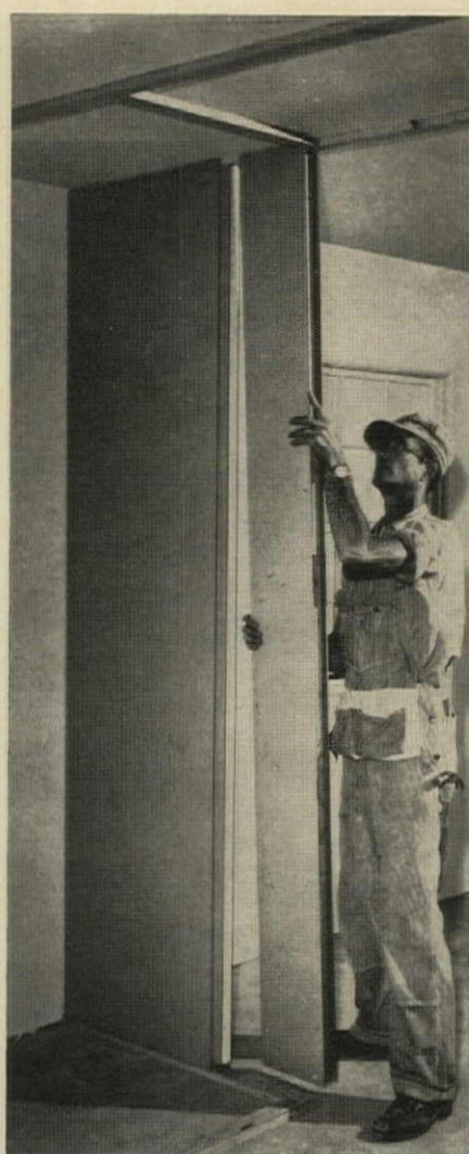
NARROW PANEL (cut to size on job) completes rear wall of closet. Exposed groove at end is closed with wood filler strip. After all partitions in house are installed, base and cove molding is added to finish job.
