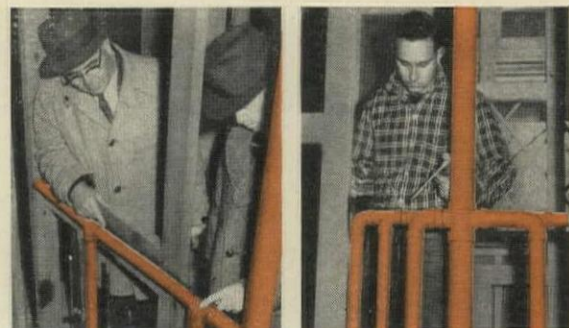
Builder James Crabb and Contractor V.J. Killian inspect Chase Copper Tube installation, made in one of two identical homes.
