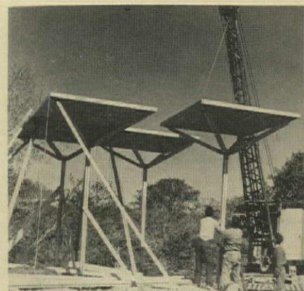
6 After fourth umbrella is set bracing is removed, other umbrellas are placed. /END
