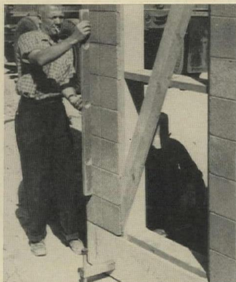
LEVELING DEVICE —a bolt-and-rod jack—is inserted in holes in grade beam to adjust panel in final position. Dry concrete is packed under beam.
