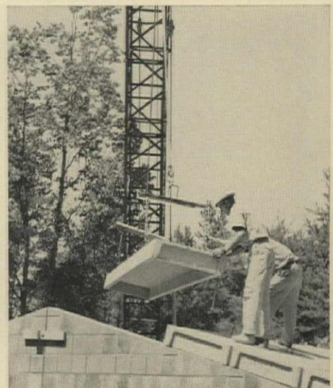
ROOF PANELS —16' or 20' long, 2'8" wide, and 8" deep—are positioned, then topped by 2x4s 24" o.c., insulating batts, sheathing, and shingles.
