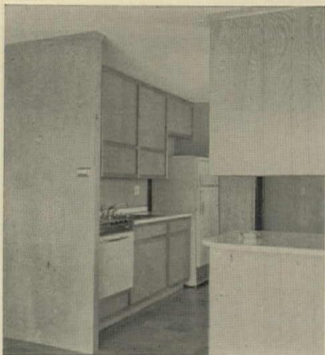
PREFINISHED CABINET DOORS and self-jigging cabinet frames (H&H, Sept.) cut kitchen costs.
