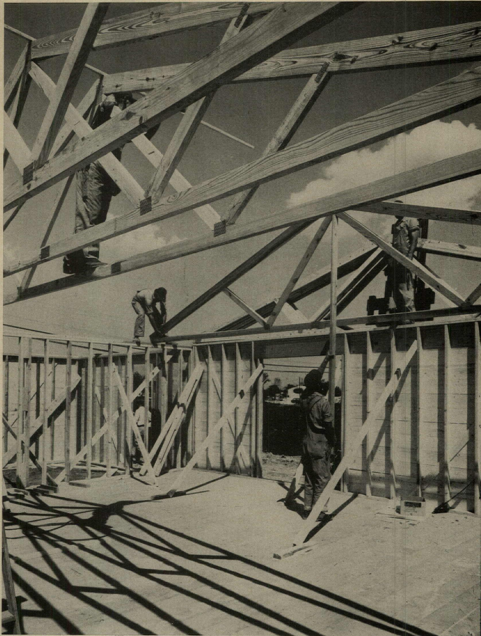
UNICOM-coded trusses, keyed to working drawings, allow quick and accurate placement on the site. W trusses eliminate load-bearing partitions for a free-span area below, too. Note use of notched gin pole for positioning.
