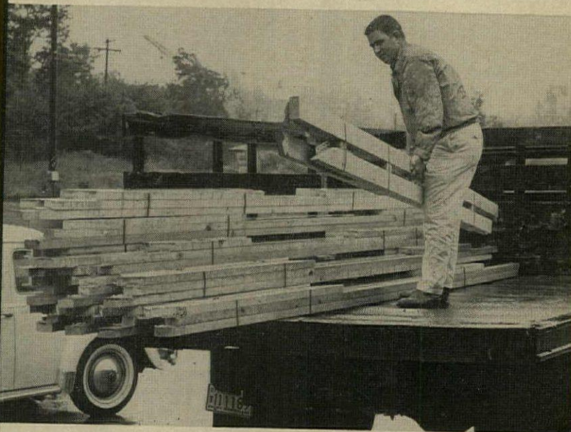
A dozen knocked down 24-foot roof trusses of West Coast Lumber occupies a small space. Trusses for several houses may be hauled in one truck load.
