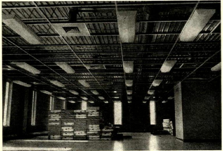
CONSTRUCTION PHOTO shows concrete floor, block walls, and bar joists that support a dropped ceiling and the steel deck for the floor above.
