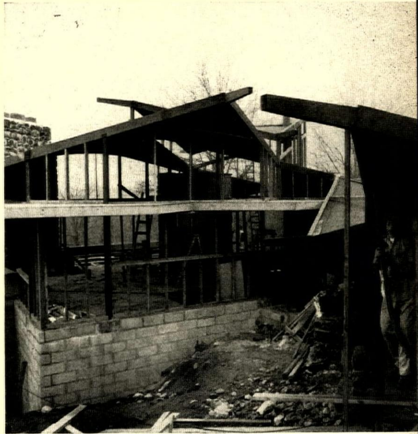
CONSTRUCTION PHOTO shows roof sections being built up with sprayed concrete before frame walls are finished.
