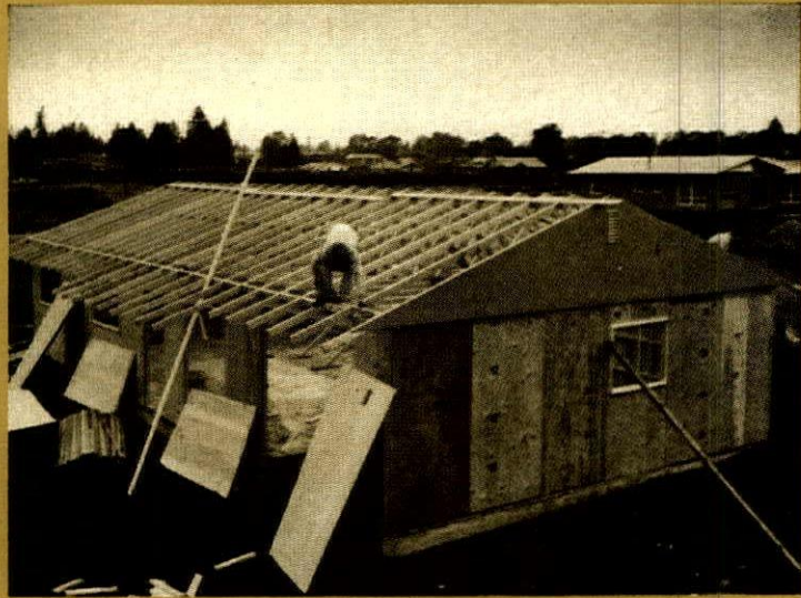
5. PlyScord roof sheathing is stacked alongside the house so the crew can reach it easily. Mayer/Peterson have never used anything but plywood for roof decking on their houses.
