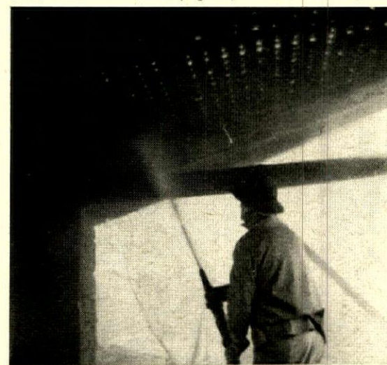
CONCRETING was done by one man. Gun has controls at nozzle, so mix could be altered as roof was built up.
