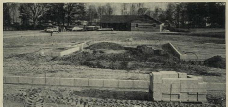
FROM FOUNDATION TO FINISHED HOUSE Schmitt is now building on site faster, more efficiently, and at lower cost because of his factory in the field.
