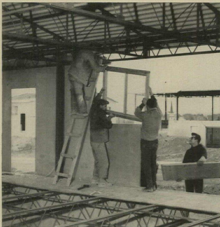
ERECTING PANEL AND WINDOW SECTION takes three men only 4½ minutes. Window channel is caulked before the section is set in place.
