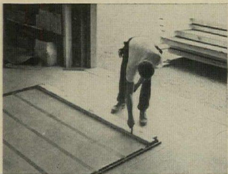
PANEL JIG is two lengths of channel iron fastened to floor, with lines marking stud spacing. Here, corner post is set into position.
