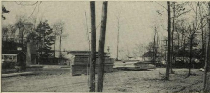
FRAMING COMPONENTS , including trusses, left , and wall panels, right , are piled next to the slab. Trusses are placed near the end of the house through which they will be carried and erected.
