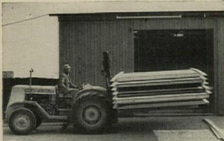
WALL PANELS are picked up at the fabricating shop door where they were piled immediately after assembly.
