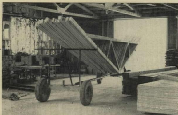
TRUSSES for one house are racked on trailer (which Schmitt built for $275) ready to be hauled to site. Boxes behind jig (left) hold gusset plates and special clinch nails.
