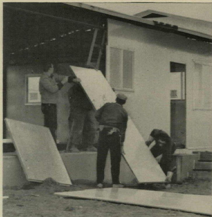
ERECTING FULL-HEIGHT WALL PANEL takes three men 3½ minutes. No steel components are too big to be manhandled on the job.
