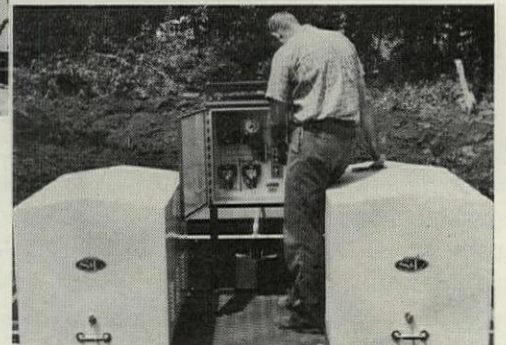
Then the treatment plant is ready for initial start-up . . .
