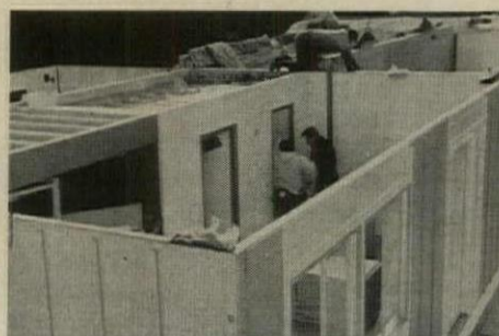
5. Walls are joined at corners by lag bolts (hole in foreground) which are covered by trim.
