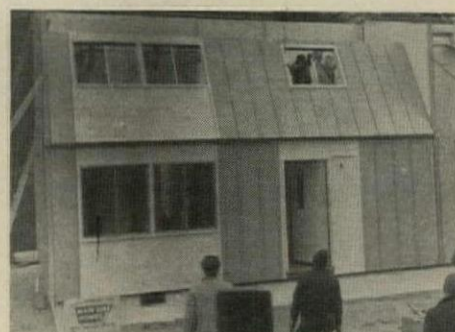
8. Upper walls are unfolded. Field-applied hinge sections tie upstairs floors to lower walls.
