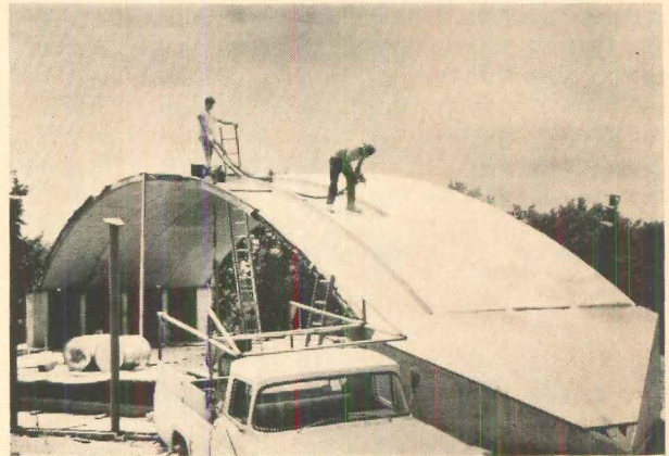
Rigid urethane, foamed in place at the job site, provides structural insulation on roof and in brick cavity walls.
