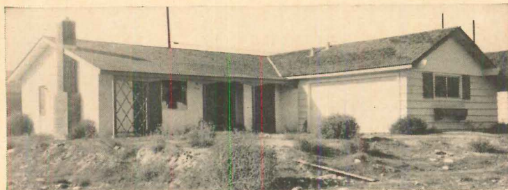
NEGLECTED FORECLOSURE has broken windows and eroded, littered yard.
