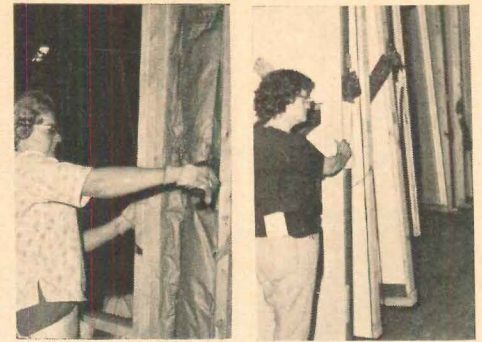
WOMEN'S WORK at National Homes includes installing insulation batts, left, and positioning wall panels suspended from a conveyor line.
