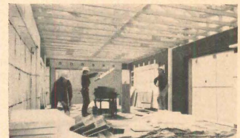
FINISH and fixtures are applied to box before it is placed. Truss-and-tarp roof is temporary.
