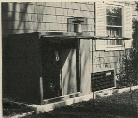
TWO-TON CHILLER —scaled down from much larger institutional equipment—makes valance cooling feasible for single-family houses. Companion boiler at right provides valance heating. Installation shown is used by Meenan Oil Co. of Hicksville, N.Y., for remodeling work.
