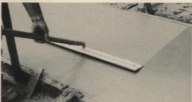
2. After screeding and tamping, the surface is smoothed with wooden floats. Final smoothing is done with this bull float. The surface is then ready for the aggregate to be seeded.
