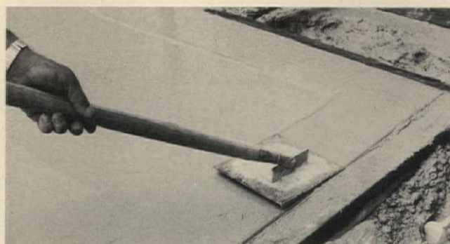
5. An edging tool is then used to secure the aggregate at the edges. This is final step before concrete sets up enough to begin the hosing and brushing operations.
