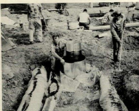
BURIED DUCTWORK includes a total return-air system that courses through an electrostatic air
