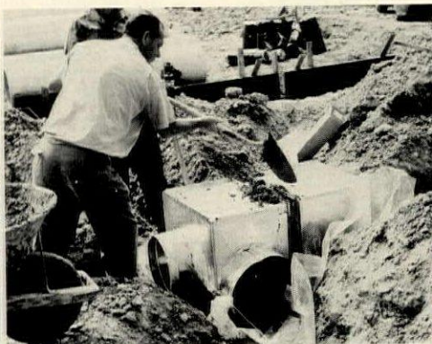
filter in buried plenum ( above ). Polyethylene wrapping keeps out water and insects.
