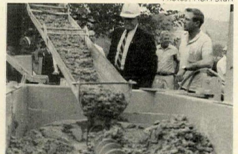
READY-MIX is distributed by auger. Paver's internal vibrators prepare cement for extruding.
