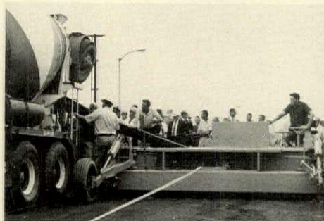
LIGHT PAVER is towed to site, then propels self on winched cable. Cement comes by truck (left).
