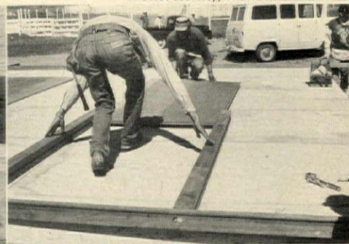
2. PLYWOOD PANEL is inserted between rabbeted studs and seated in rabbeted bottom plate.
