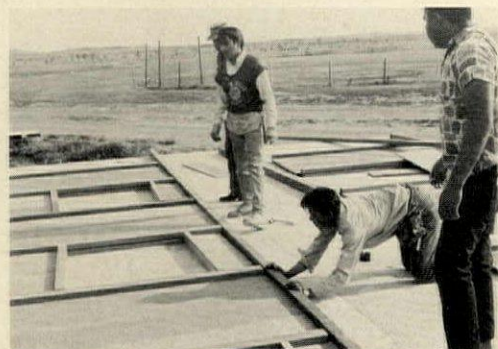
3. TOP PLATE , predrilled and rabbeted, is attached after plywood and window framing are set.
