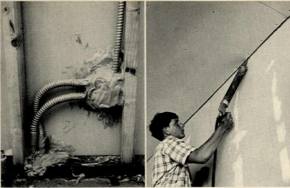
paths between walls—e.g. (left to right), wood-frame joints, electrical-box holes and wall seams.
