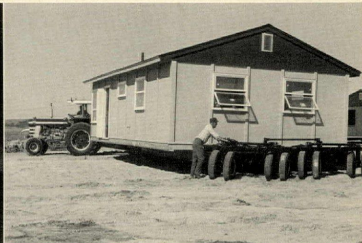
HYDRAULIC TRAILER with rear steering lifts house off assembly-line chassis ( left ) and lowers it onto precast foundation at the building site.
