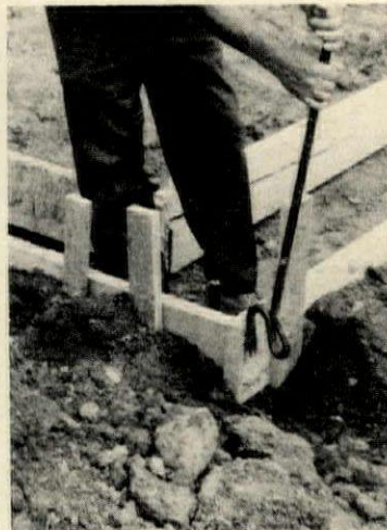
10 Modified crowbar speeds nail pulling. When disassembling forms and scaffolding, laborers used to pull nails with an ordinary carpenter's hammer, which required bending and stretching.
