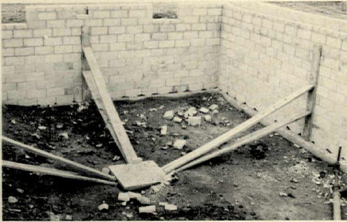
7 Bracing ends wall buckling, cuts down on hairline cracks. Half of Meyerhoff's houses used to need foundation-wall repairs
