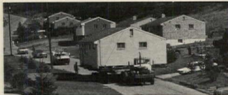
HOUSE MOVING is part of Pittsburgh builder Pat Minnock's business. He bought 21 slated for demolition, moved them and rented them out.
