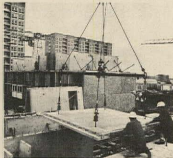
Floor slab with projecting loops is lowered into position over threaded tie-bolts in ground-floor walls.
