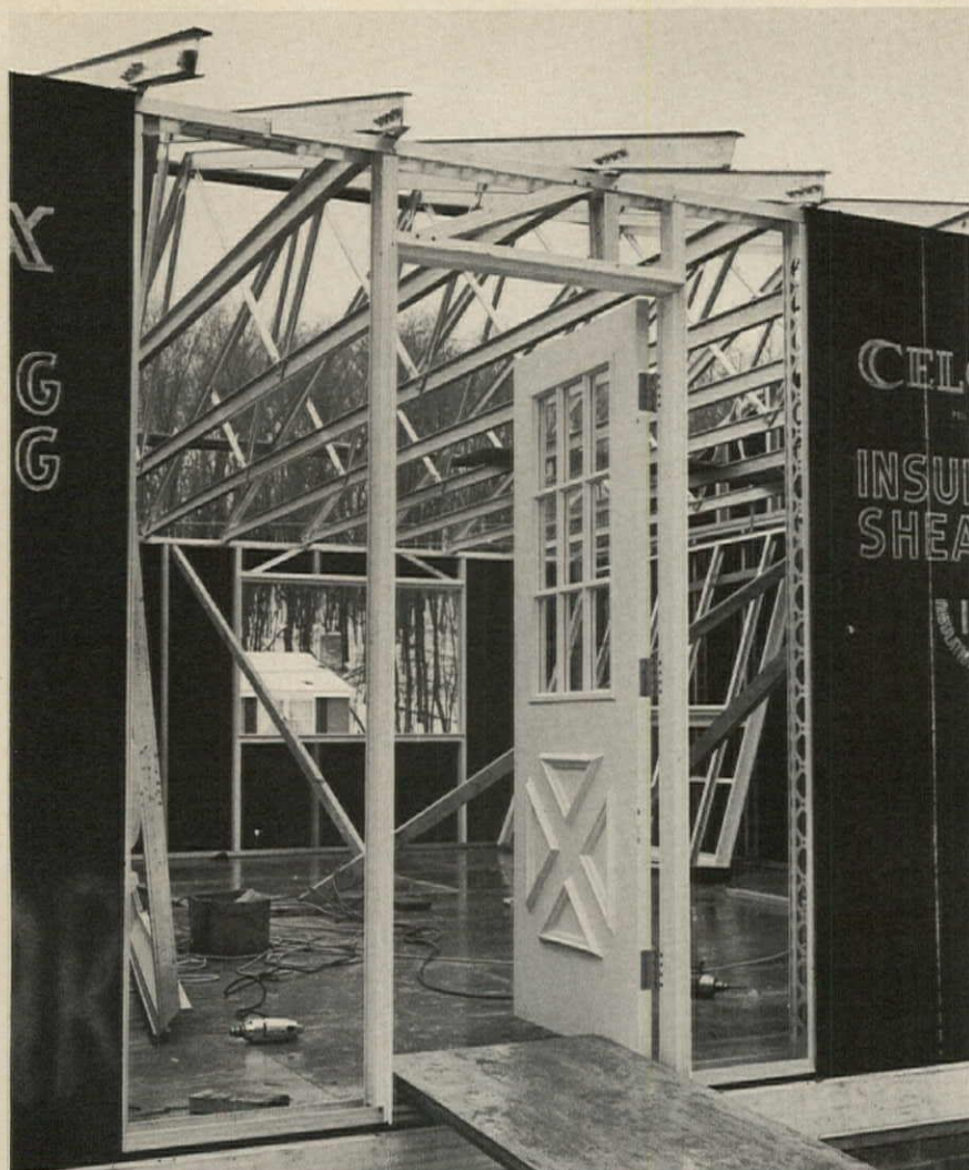
Aluminum door frame has fewer parts than wood frame, is factory-painted. Both the trusses and the prepunched studs are set on 24" centers.
