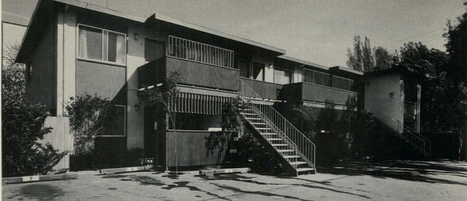
Balconies and terraces (above) were added to the plain-Jane apartment building (below, right) in a relatively simple fix-up procedure. Results: an increase in monetary as well as aesthetic value, and more privacy from the street for tenants. New grilles block out view of cars and pavement from apartments.
