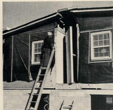
End wall is closed in with a 3' x 8' prefabbed panel. Floor joist fillers have already been installed, but in this photo roof is not yet raised.
