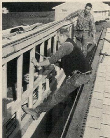
New kneewall section is inserted between small kneewall and roof stringer. Jacks have been removed, and roof rests on new wall.
