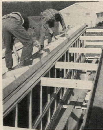
Collar beams are nailed between kneewalls, and half of the new roof structure is prepared. Shingles and cap will then be put on.
