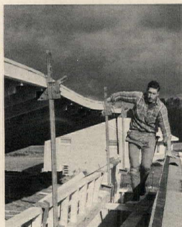
Roof is jacked up from position in which it was shipped (photo, above) to create 4-in-12 pitch. Small kneewall supported roof in transit.
