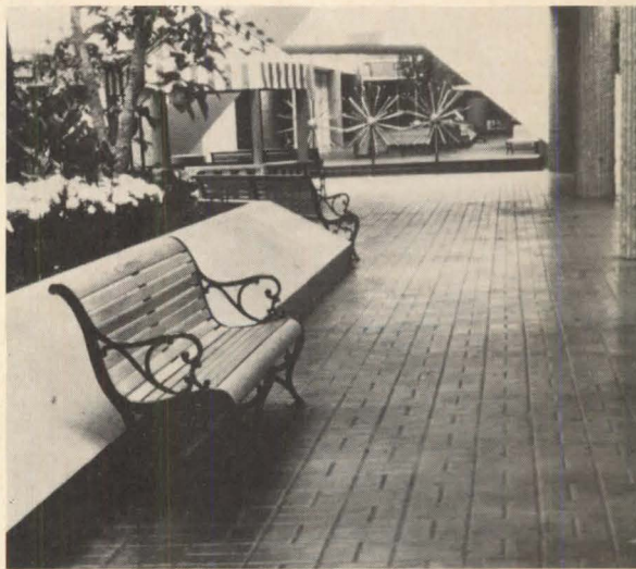
"Thinset" concrete topping (above) is poured over concrete slab. The topping, primarily used for retrofit applications, may be formed in a variety of patterns according to the template used. Bomanite, Palo Alto, CA. Circle 262 on reader service card
