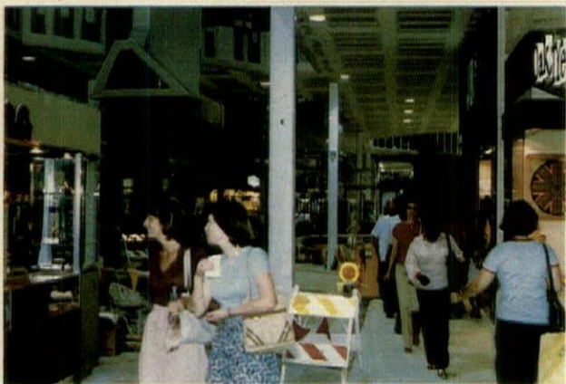
Business as usual. Daytime shopping continued while Sharps-town Mall was updated at night. Note workers removing roof by hand because old structure couldn't handle heavy machinery.
