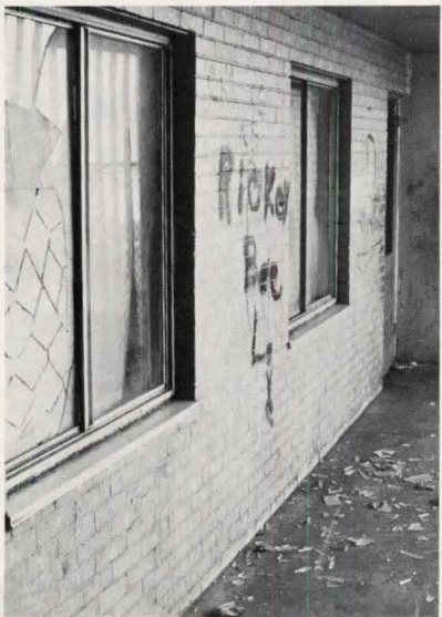
Deficient management, leading to project deterioration like that shown above, is one charge leveled at CHA.
