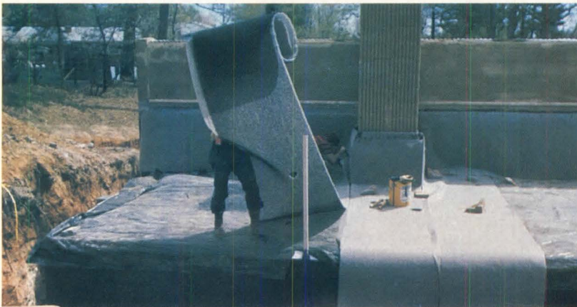
Lightweight 'Enkadrain' matting relieves the hydrostatic pressure build-up that may occur in soil that drains poorly. Composite matting, shown being installed on the roof of an earth-sheltered residence, consists of a compression-resistant nylon mesh webbing heat-bonded to a polyester fabric. Protective matting comes in rolls 99' long and 38' wide. American Enka Company. Circle 266 on reader service card
