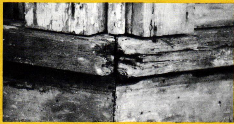
This rotted – and irreplaceable – woodwork...
