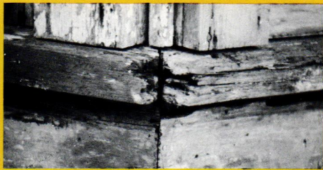
This rotted – and irreplaceable – woodwork...
