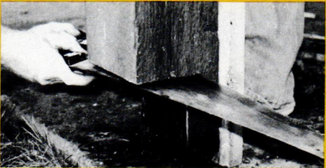
10" rotted bottoms of these load-bearing columns...
