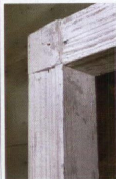
ABOVE: The stabilized Huff-Blalock House, which dates to 1815, has 12" to 15" wide planking on walls and ceilings. LEFT: A moulding detail on a door casement.
