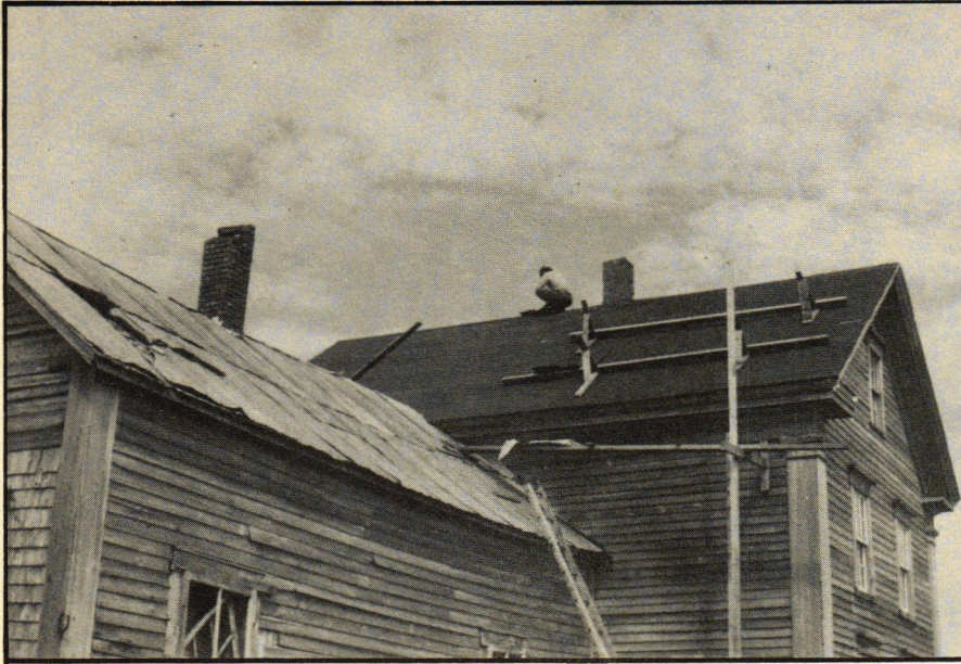
Ell in the foreground shows the condition of the siding and roof that confronted the Ryans. Danny rigged a scaffold for re-roofing the main section of the house.
