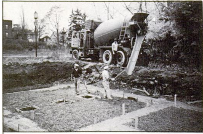
Meanwhile, at the new site, footings are being poured and crushed stone brought in.
