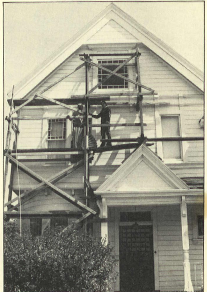
Peter and Jean climb the scaffolding at the outset of the restoration. Old paint and scars from the original wood trim helped them to mount the redwood replacements.
